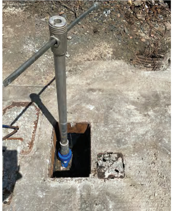
A VIDI Positioner installed in-situ underground.
